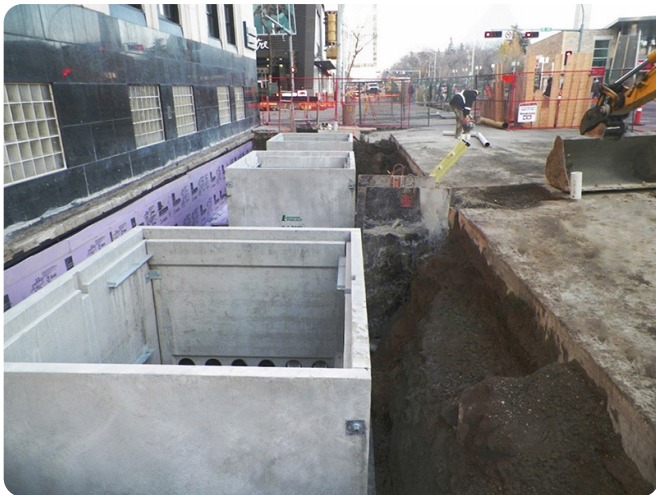
Composite trench covers provide better protection against harsh weather elements year-round
